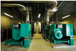
Power Generation and Distribution Systems
