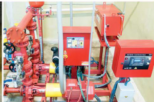
Fire Protection Systems
